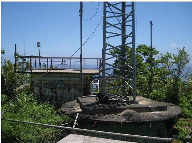
Figure 9. Radio tower and equipment storage.
